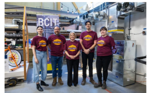
Minister of Post Secondary and Future Skills Lisa Beare visit the BCIT Residential Heat Pump Lab
